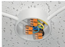
Lighting distribution in a ceiling canopy
