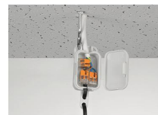
Pendant light connection in a suspended ceiling
