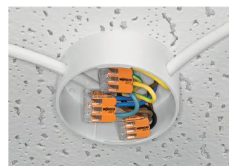
Lighting distribution in a ceiling canopy
