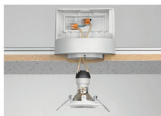
Custom low-voltage lighting system
